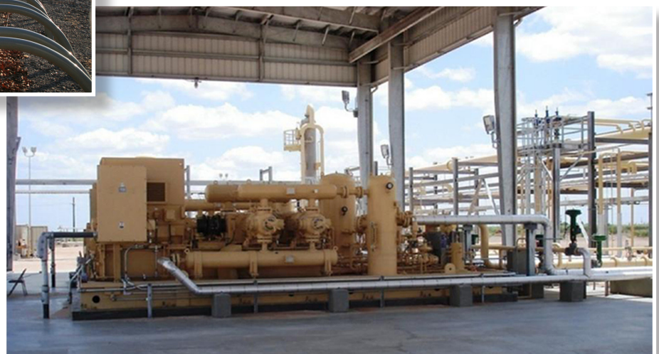
Compressor for compressing gas prior to re-injection
