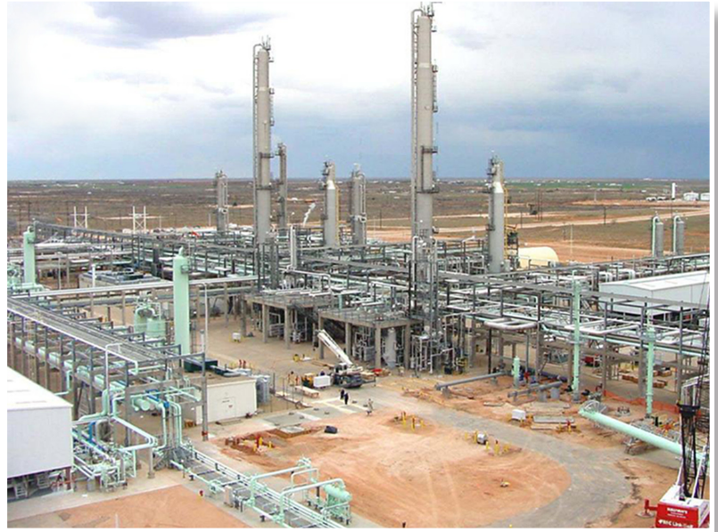
CO 2 processing plant where the gas is collected for re-injection
