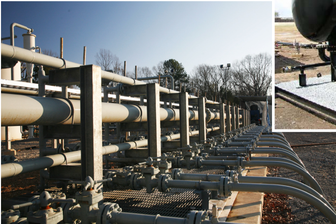
Well production manifold to allow individual testing of wells
