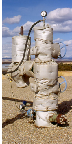
Insulated CO 2 source wellhead
