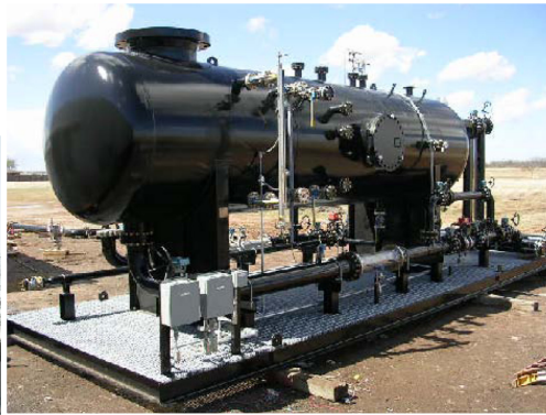
Separator for separating produced fluids (oil, water, and gas)
