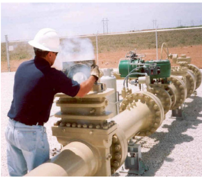
CO 2 pipeline metering
