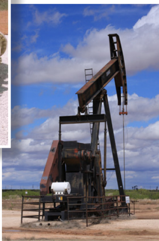
Production well pump jack
